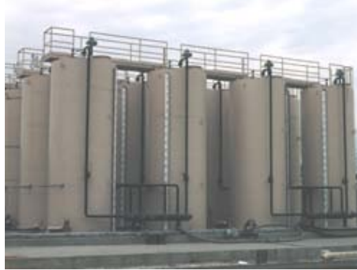
Bulk Storage Silos & Tanks
