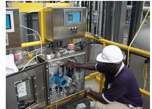
Vent Header Monitoring
